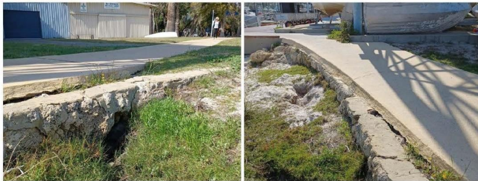
Figure 3.21 Undermined Limestone Block Wall
