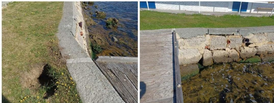
Figure 3.23 Deteriorated Limestone Block Wall
