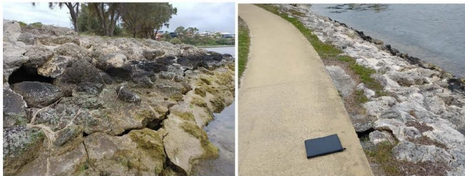
Figure 3.12 Grouted Revetment (L) & Voids Under Path (R)
