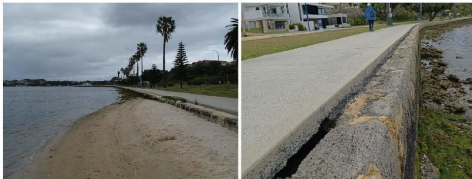
Figure 3.8 Low Limestone Blockwall (L) & Voids Beneath Path (R)
