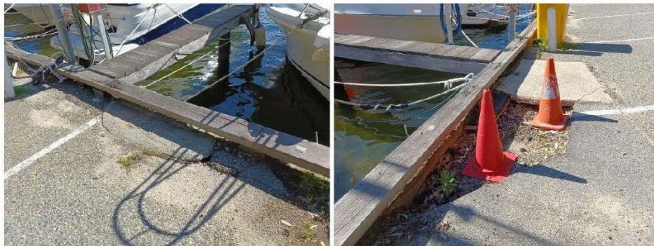
Figure 3.31 Carpark Bitumen Repairs & Settlement
