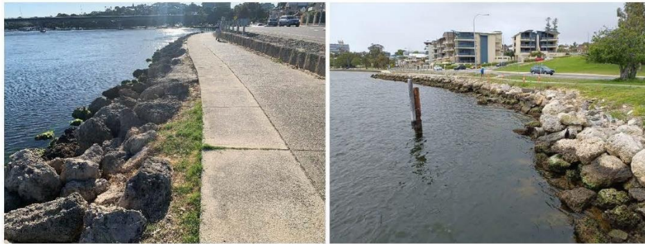
Figure 3.1 Path Behind Revetment (L) & Overtopping Damage (R)
