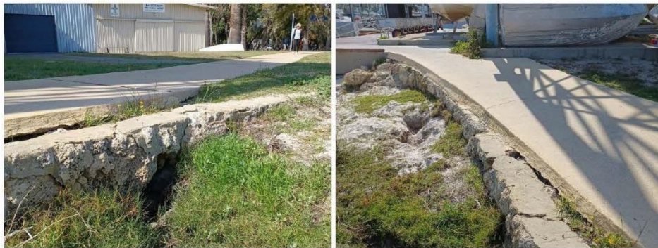
Figure 3.21 Undermined Limestone Block Wall
