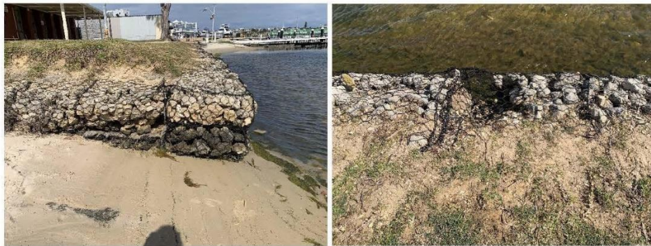
Figure 3.18 Limestone Gabions Rotated (L) & Lost Material (R)
