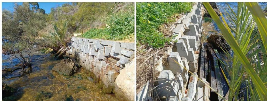
Figure 3.24 Deteriorated Crib Wall
