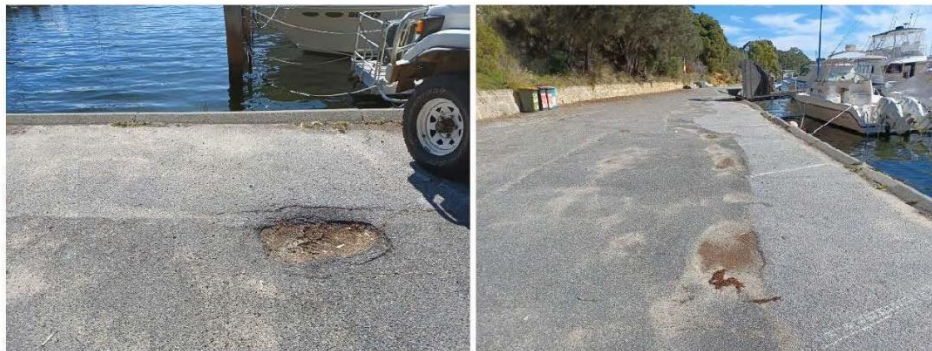
Figure 3.29 Carpark Pot Holes & Repairs
