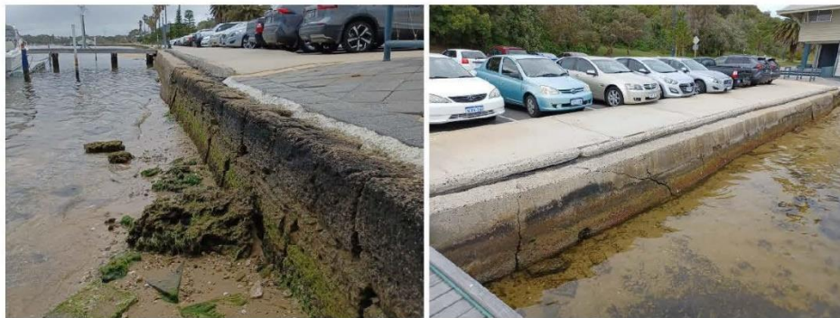
Figure 3.7 Weathered Blockwall (L) & Cracking of Concrete Wall (R)
