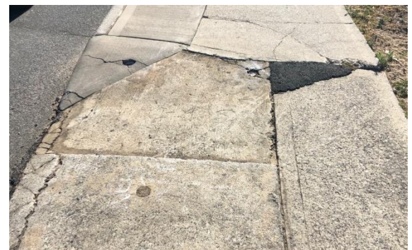
Cracked pavement repaired but uneven
