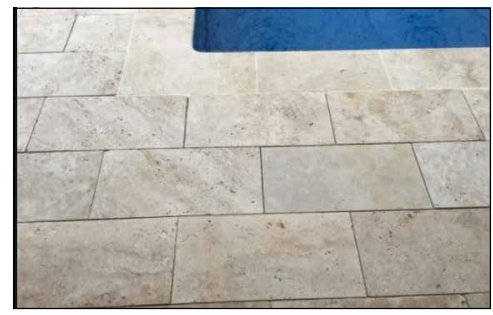
TRAVERTINE PAVING LAID IN STRETCHER BOND PATTERNS AS PER PICTURE ABOVE PAVING AREAS: TOTAL BELOW 228sqm EXCLUDING OFFCUTS - FRONT PORCH AND SIDE OF HOUSE DOWN TO LAUNDRY - SIDE OF GARAGE AND STORE INCLUDING STAIRCASE DOWN - LOWER GROUND FLOOR SITTING AREA AND RAMP DOWN TO POOL - POOL AREA INCLUDING POOL AREA STAIRCASE
