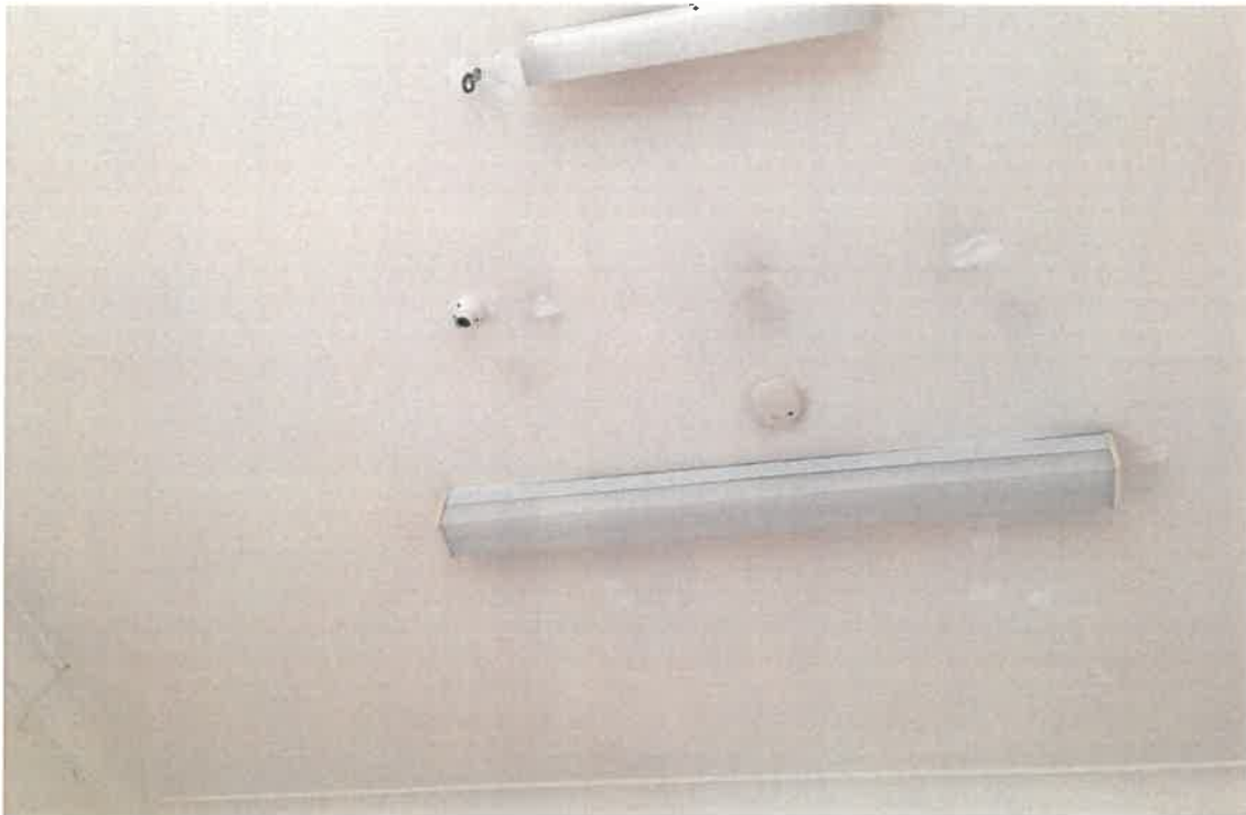
Image 18: Miscellaneous electrical fittings to be removed in ceilings throughout, image taken by DPLH October 2017.
