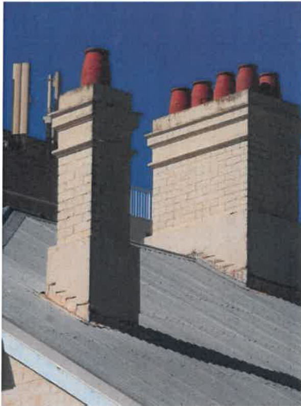
Image 13: Dilapidated chimney flashings to be replaced, image taken by DPLH October 2017.
