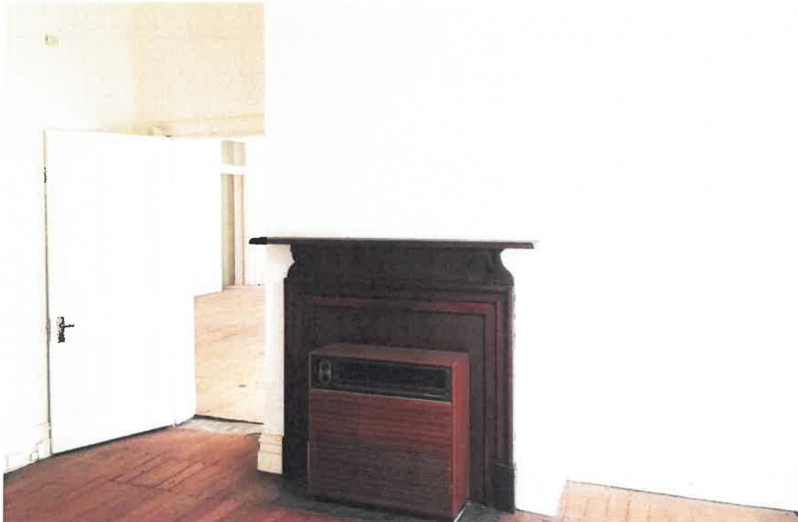
Image 21: Later addition heaters and hoardings to be removed from all fireplaces, image taken by DPLH October 2017.
