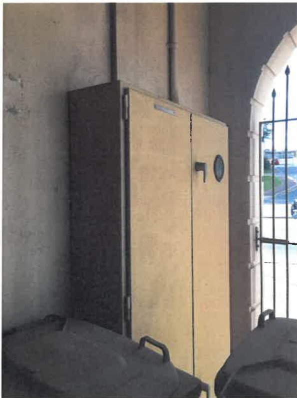
Image 14: Site main switchboard to be reduced in size, and the asbestos backing board removed, image taken by DPLH October 2017.
