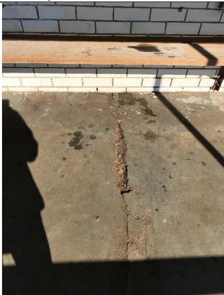
Photo 17-5-19, 11 07 06 am • Cracks along the concrete pavement. Recommend a structural topping screed is installed with a paint finish.
