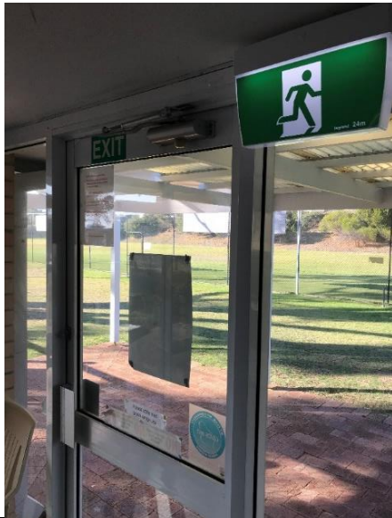
Photo 17-5-19, 8 53 29 am • Internal snib locks to exit doors do not comply with current requirements – these should be replaced with lever action locks / handles. • Illuminated exit sign is not in the correct location.
