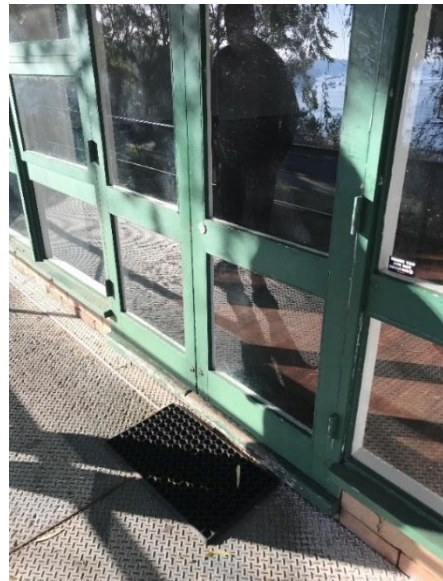
Photo 17-5-19, 8 32 52 am • Timber windows / doors to be stripped back (paint), puttied up, primed and painted.
