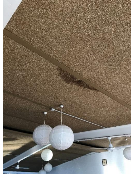
Photo 17-5-19, 8 34 00 am • Vermiculite type ceiling to hall area is in relatively good condition, some area indicating water damage.
