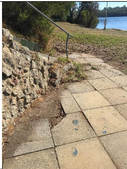
Photo 17-5-19, 11 03 43 am • Cracked and broken concrete paving. Recommend lifting the paving and relaying pavers to remove trip hazards.
