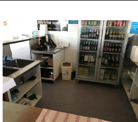
Photo 17-5-19, 8 52 49 am • Vinyl flooring has a void patch underneath the bin for the floor hatch. Recommend replacing existing the floor vinyl.
