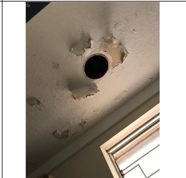
Photo 17-5-19, 9 39 26 am Paint to the ceiling is peeling, possibly caused by water. Recommend investigating roof leak and replacing ceiling.
