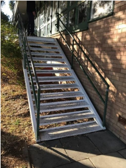
Photo 17-5-19, 8 32 06 am • Steel access stairs, platform and treads are closed chequer plate. A non-slip treatment is recommended if the stair is to be retained.
