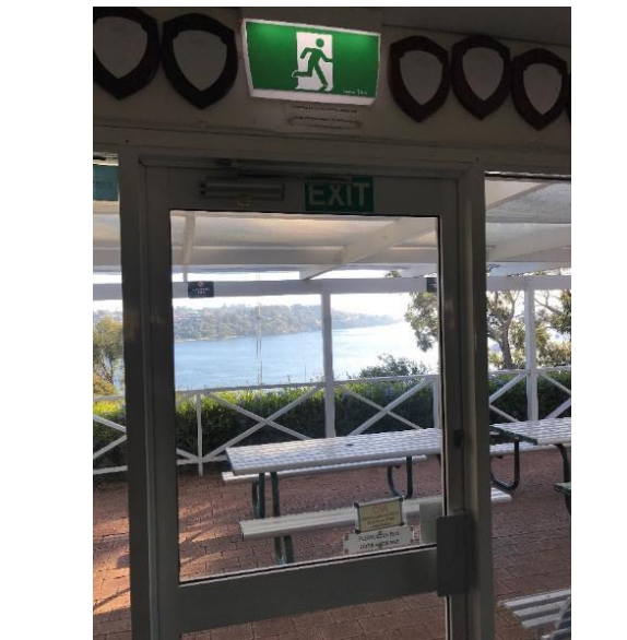
Photo 17-5-19, 8 53 13 am • Internal snib locks to exit doors do not comply with current requirements – these should be replaced with lever action locks / handles.
