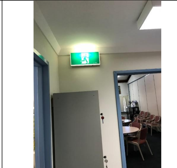
Photo 17-5-19, 9 37 55 am Exit signage strategy does not appear to be compliant – example signage to corridor requires to be directional rather than indicating that the exit direction is straight on.
