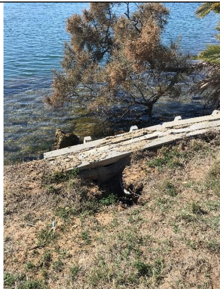
Photo 17-5-19, 11 11 44 am • Large hole with exposed service underground. If this service requires to be accessible recommend installing a pit over it and backfilling the hole.
