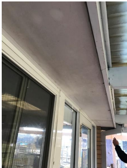
Photo 17-5-19, 8 54 31 am • Rusting evident to the soffit of the gutter / fascia. Treat the rust and paint/protect the surface including eaves.
