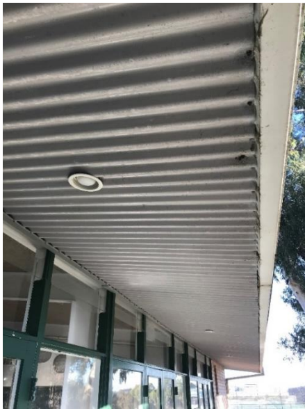
Photo 17-5-19, 8 33 14 am • Light fittings to the soffit are dropping. These should be reset and secured. • Rusting evident to the soffit of the gutter / fascia. Treat the rust and paint/protect the surface.
