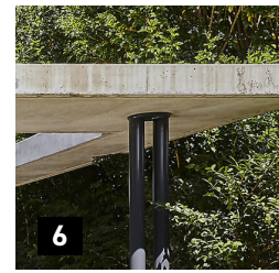
OFF FORM CONCRETE
