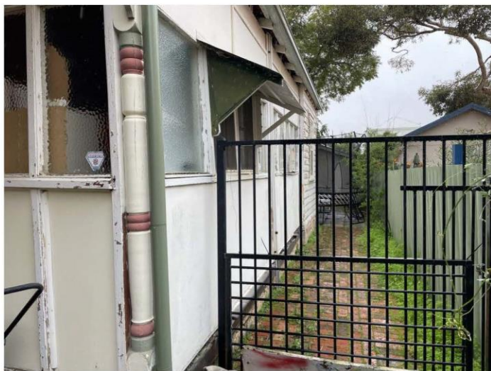
Photograph 4 The early timber addition to the rear and the more recent one in the foreground. Griffiths Architects July 2022 Some verandah posts remain and others may be concealed by the cladding.
