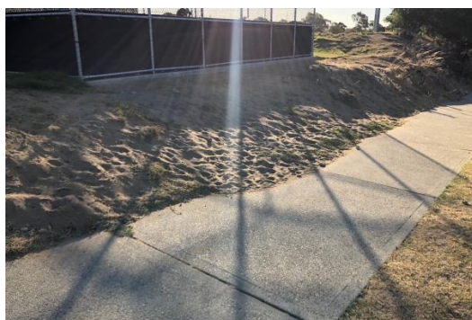
Sand on pathways – needs treatment to retain
