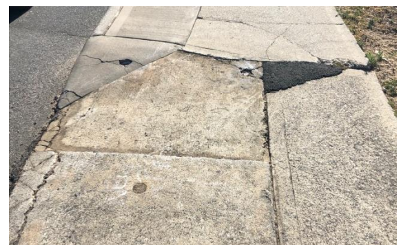
Cracked pavement repaired but uneven
