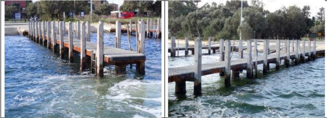
All chaffers are in place and secured. (24 chaffers per jetty, 48 in total)
