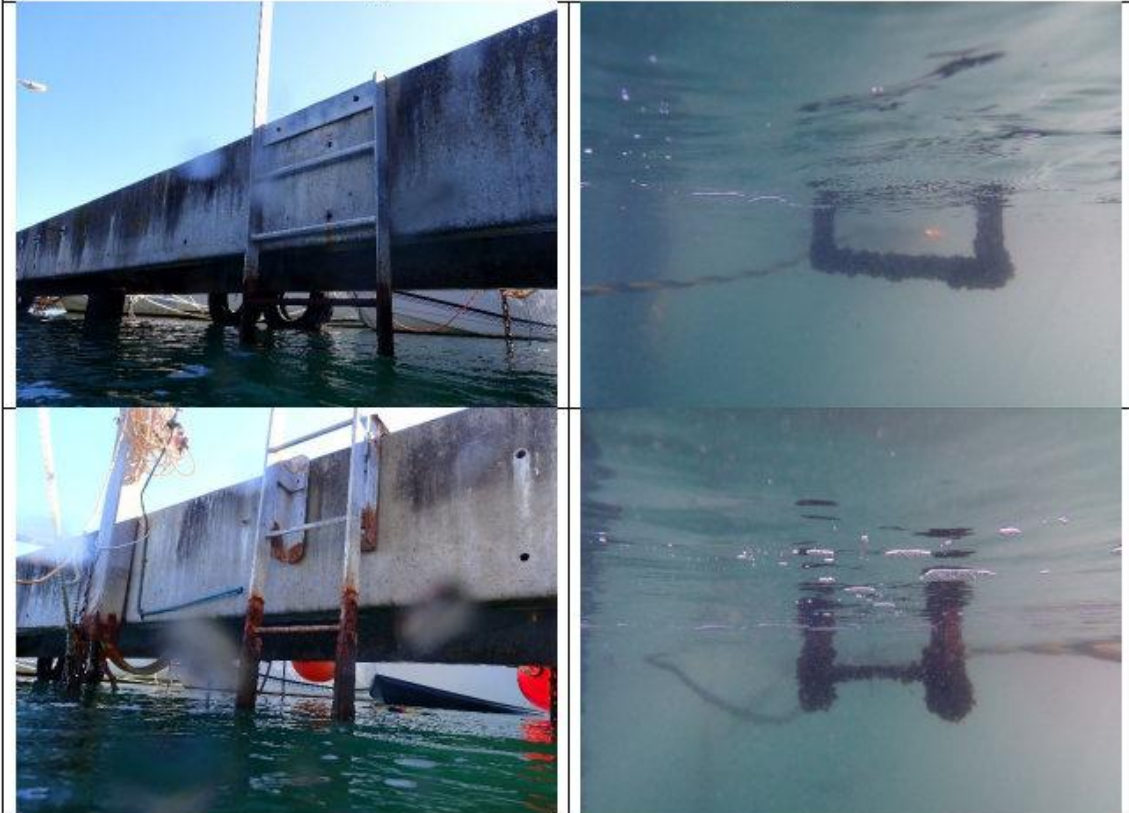
Two mild steel ladder appears to be in fair condition with rust present at water level
