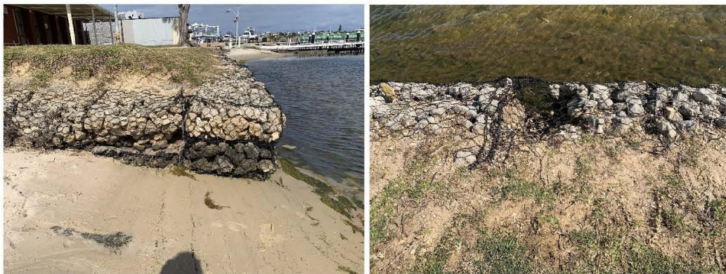
Figure 3.18 Limestone Gabions Rotated (L) & Lost Material (R)
