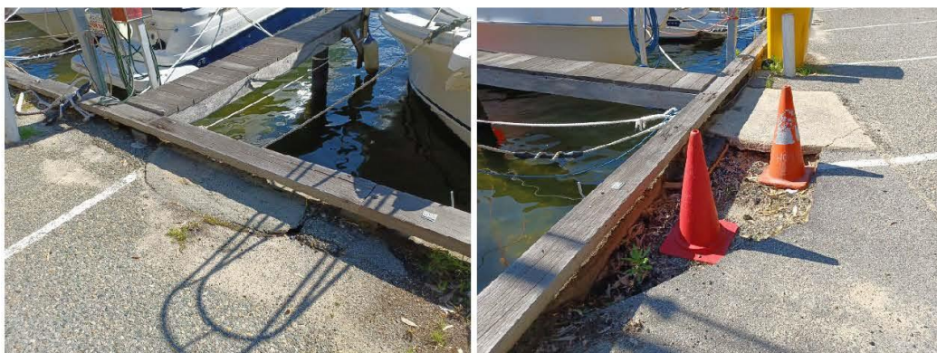
Figure 3.31 Carpark Bitumen Repairs & Settlement
