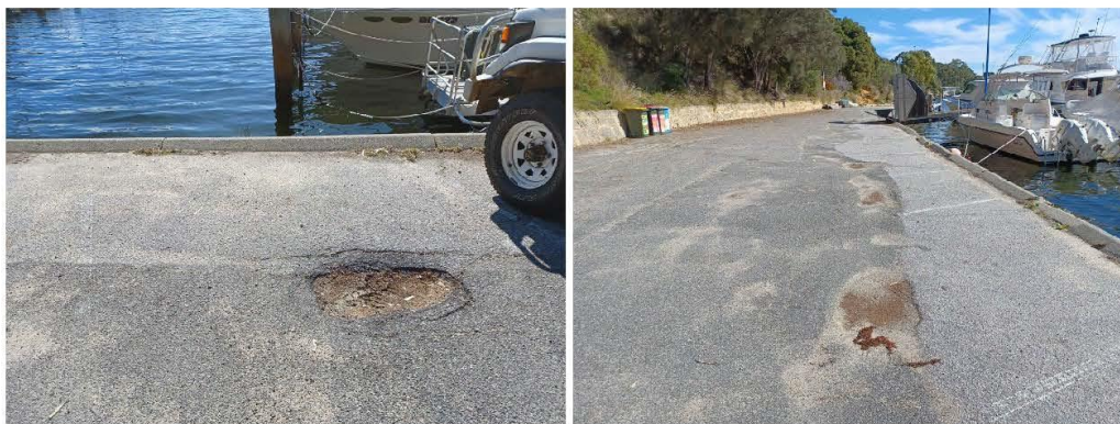
Figure 3.29 Carpark Pot Holes & Repairs
