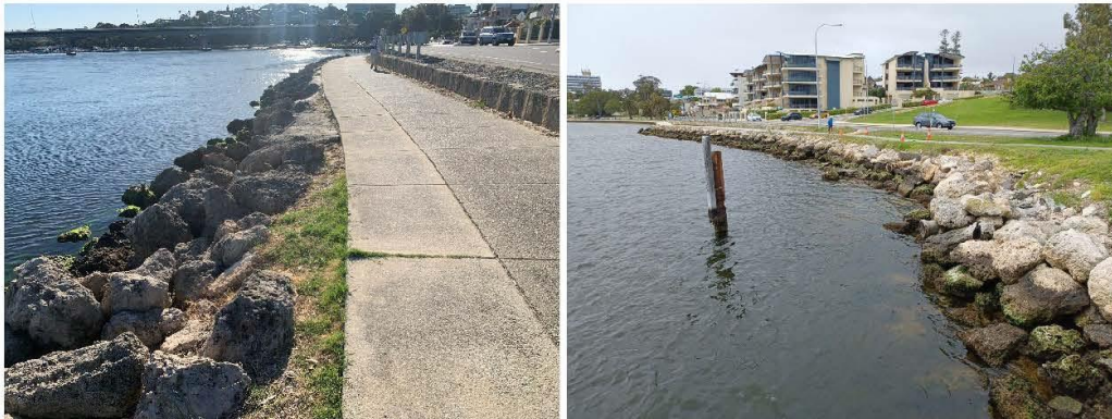
Figure 3.1 Path Behind Revetment (L) & Overtopping Damage (R)
