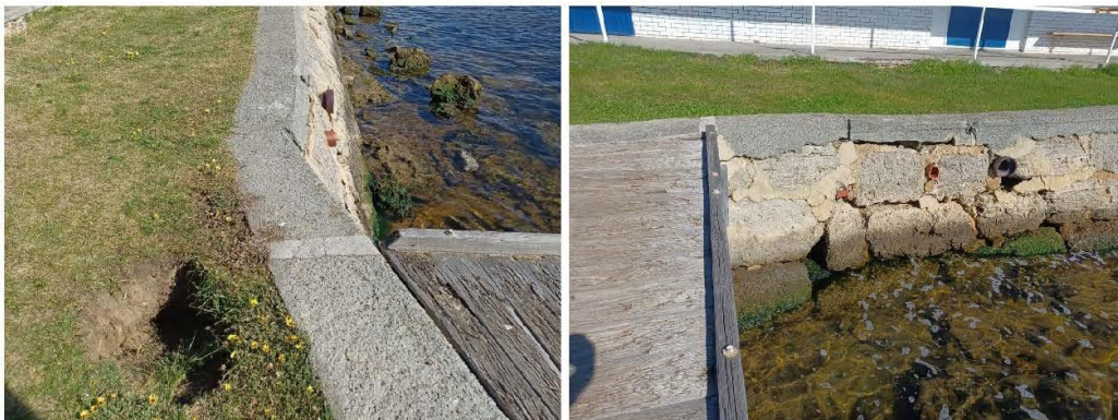
Figure 3.23 Deteriorated Limestone Block Wall
