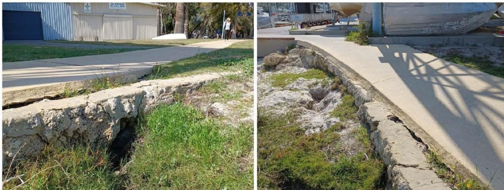
Figure 3.21 Undermined Limestone Block Wall
