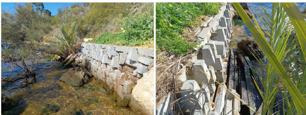
Figure 3.24 Deteriorated Crib Wall
