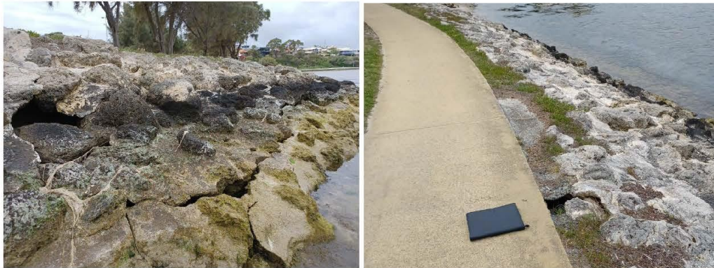
Figure 3.12 Grouted Revetment (L) & Voids Under Path (R)
