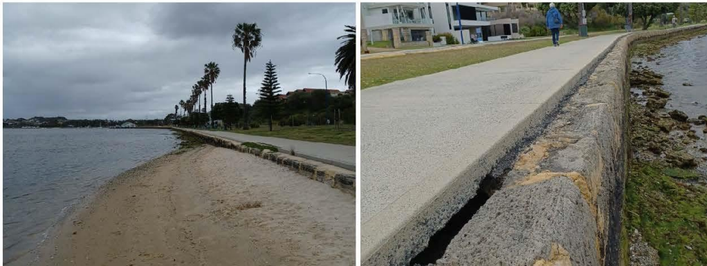
Figure 3.8 Low Limestone Blockwall (L) & Voids Beneath Path (R)
