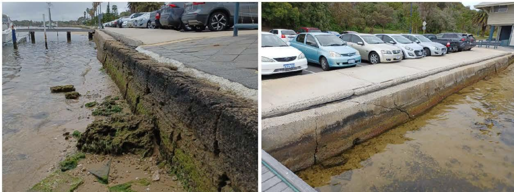
Figure 3.7 Weathered Blockwall (L) & Cracking of Concrete Wall (R)
