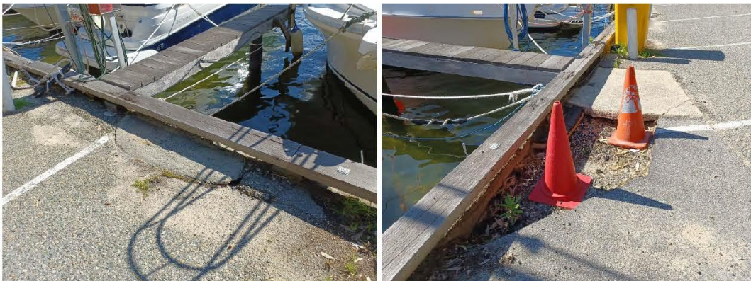
Figure 3.31 Carpark Bitumen Repairs & Settlement
