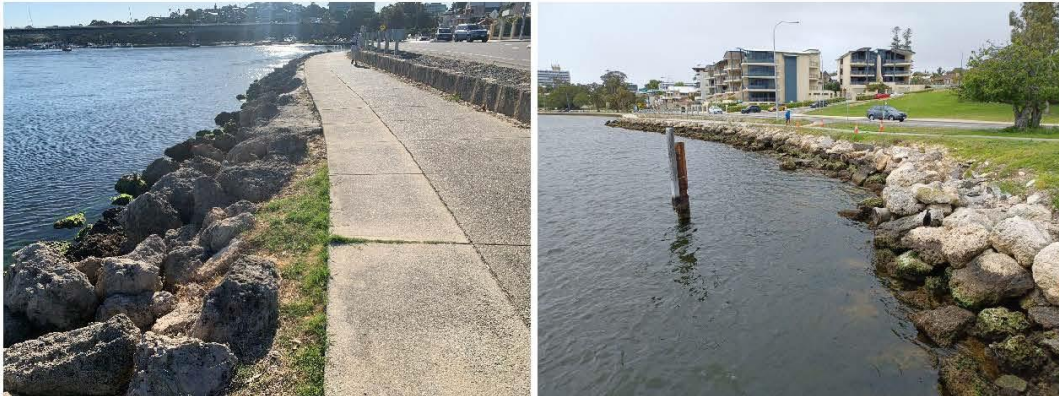
Figure 3.1 Path Behind Revetment (L) & Overtopping Damage (R)
