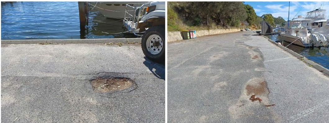
Figure 3.29 Carpark Pot Holes & Repairs
