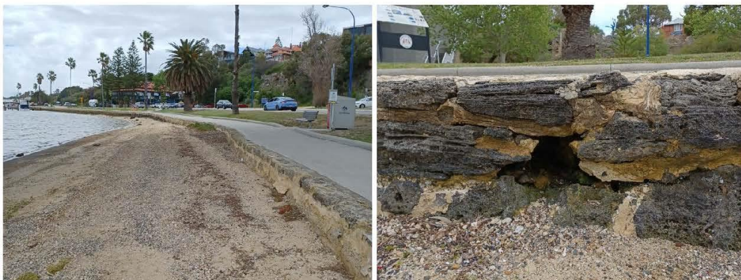
Figure 3.4 Sandy Beach (L) & Downstream Void (R)
