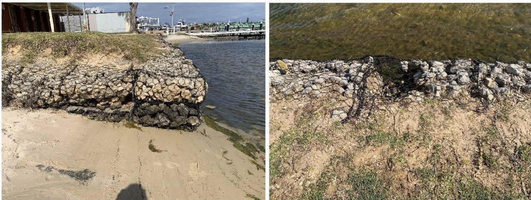
Figure 3.18 Limestone Gabions Rotated (L) & Lost Material (R)
