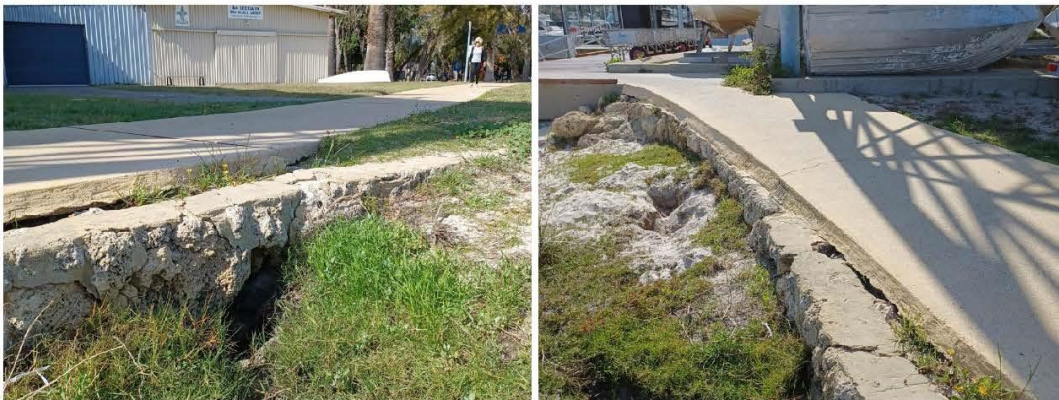
Figure 3.21 Undermined Limestone Block Wall
