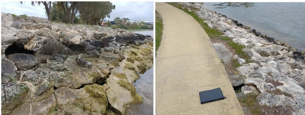
Figure 3.12 Grouted Revetment (L) & Voids Under Path (R)
