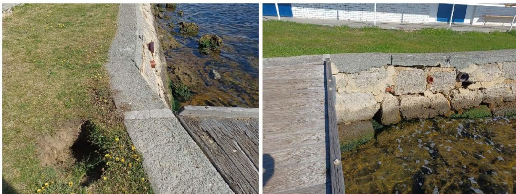
Figure 3.23 Deteriorated Limestone Block Wall
