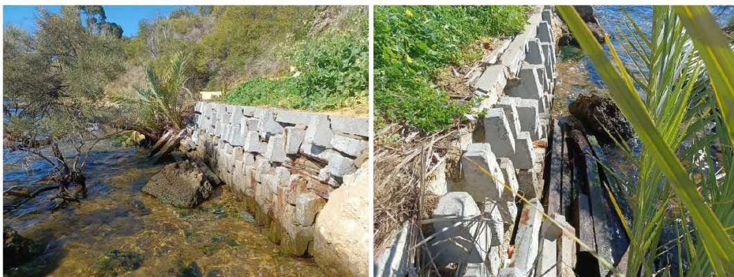
Figure 3.24 Deteriorated Crib Wall
