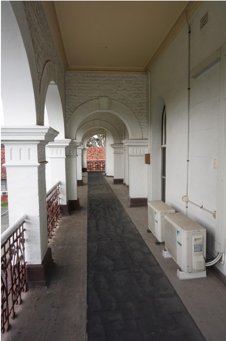
Photo 08 First floor verandah looking east. The malthoid flooring was a later addition. The condensers will be removed.
