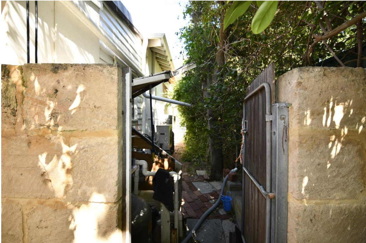
Photo 12 The original north wall to the house has been rendered.
