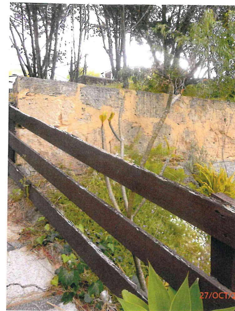
Solid retaining wall dividing 50A View Tee & top verge. Above this can be seen the brick foundations on which the old wooden bus shelter near Bus Stop 11079 on Upper View Tee
