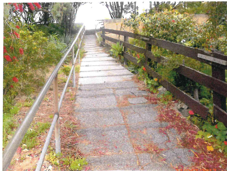
Going up ramp. Dilapidated, splintered post and rail fence seems to be E boundary of 50A View Tee
